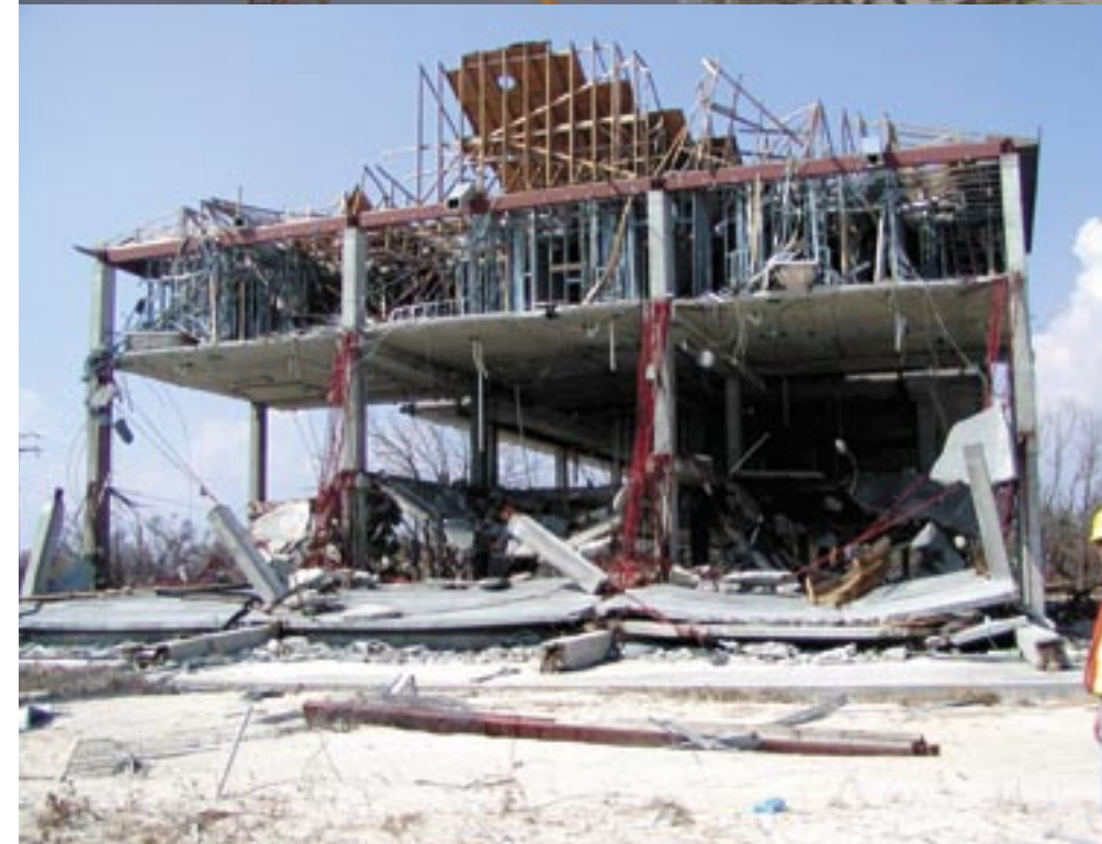
The casino of the Hard Rock Hotel & Casino Biloxi was built on floating pontoons enclosed in a fixed exterior structure. Collapse of the entire structure, top, is thought to have resulted from pounding between the pontoons and the inland columns supporting the exterior structure. Hydrodynamic uplift of the posttensioned flat slab in the bay closest to the shoreline appears to have initiated the frame collapse of a concrete building frame under construction on U.S. 90 in Pass Christian, Mississippi, above.
