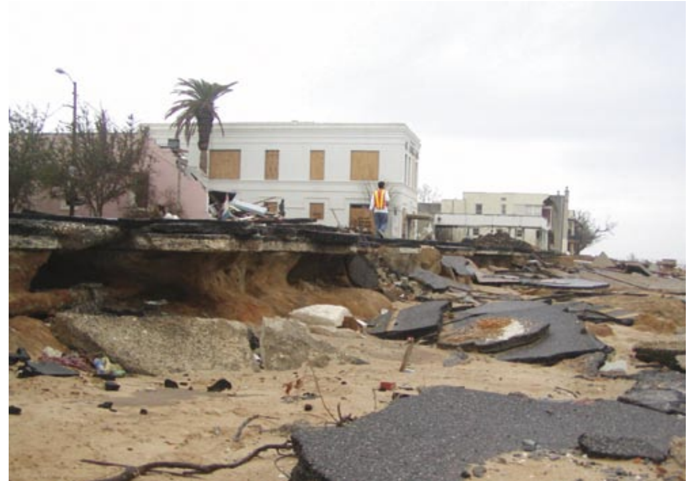
The complete failure of North Beach Boulevard—the coastal highway through Bay St. Louis, Mississippi—was due to a combination of liquefaction and shear-induced scour.
