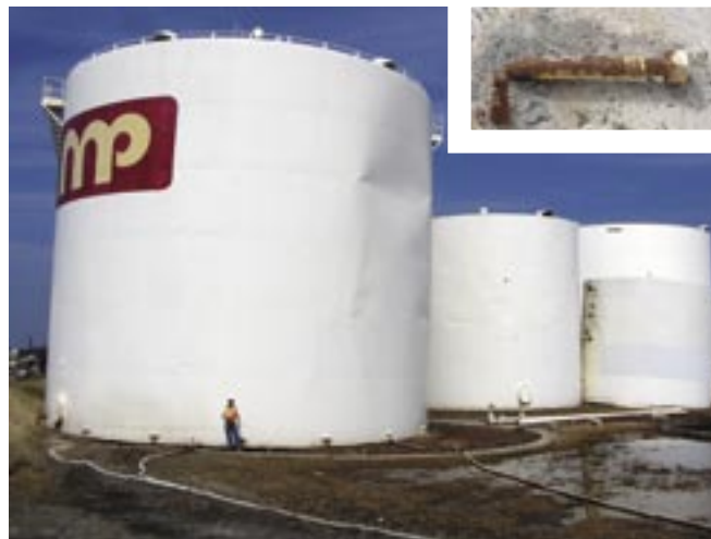
The storm surge exceeded the elevation of the containment berm surrounding a series of fuel storage tanks at Rhodes Point, in Biloxi, Mississippi. Buoyancy of the empty or partially empty tanks resulted in failure of the corroded anchor bolts, inset.
