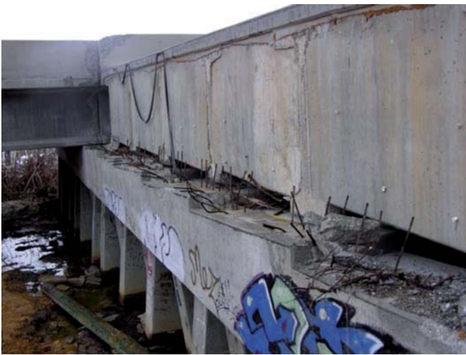
Figure 9. Inadequate dowels at bent support.
