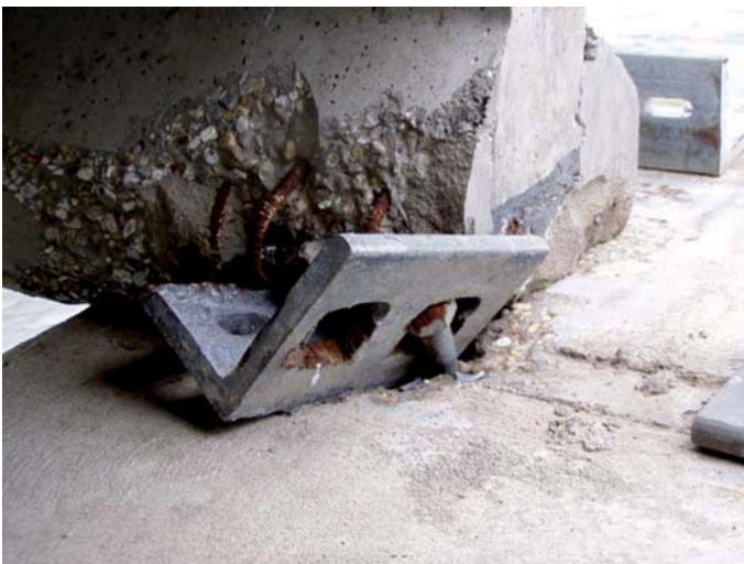
Figure 15. Failure of restraint due to flame cut oversized hole.
