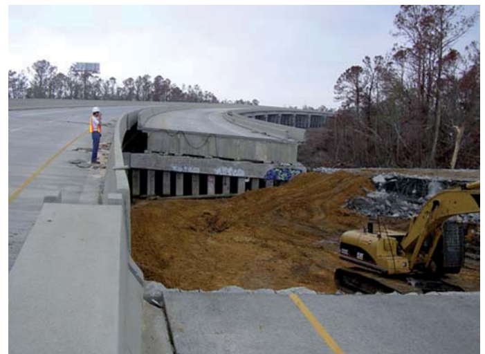
Figure 7. Single span of US90 washed from supports.
