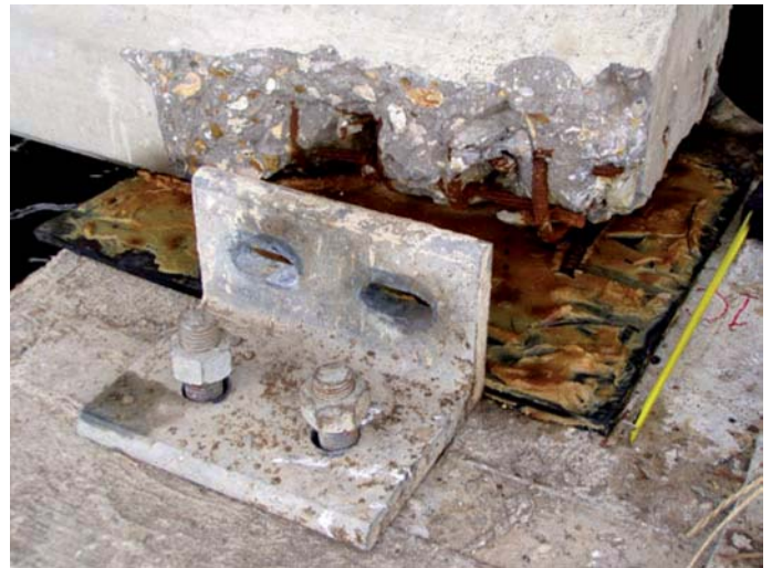
Figure 12. Failure of restraint due to anchor bolt pull-out.
