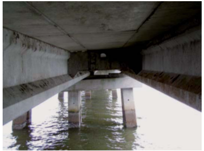
Figure 11. Reduced bridging and holes to allow airflow.
