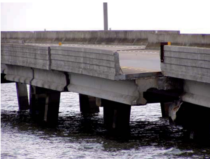
Figure 10. Dislocated segments of I-10 onramp, Mobile, AL.
