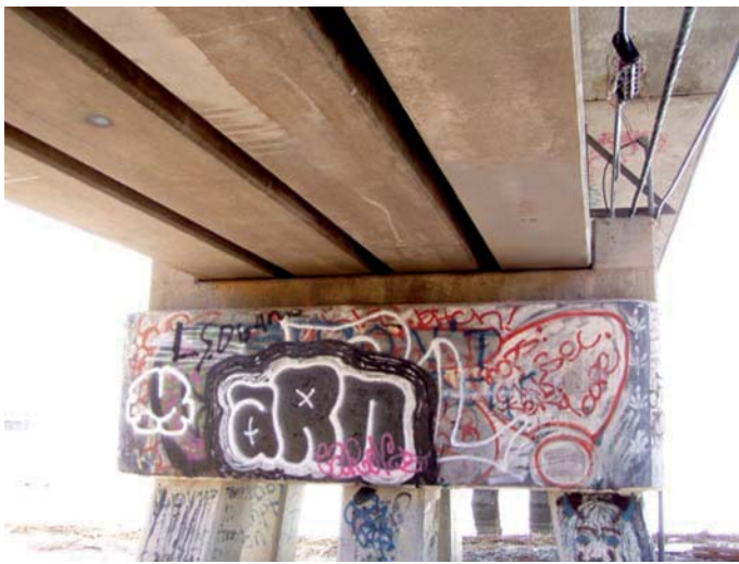
Figure 18. Large concrete shear keys on either side of closely spaced railroad bridge girders.
