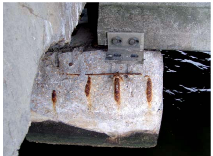
Figure 13. Failure of restraint due to anchor bolt edge spall.
