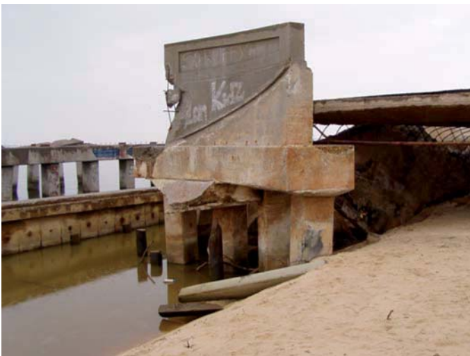
Figure 6. Scour around abutment and under approach slab.
