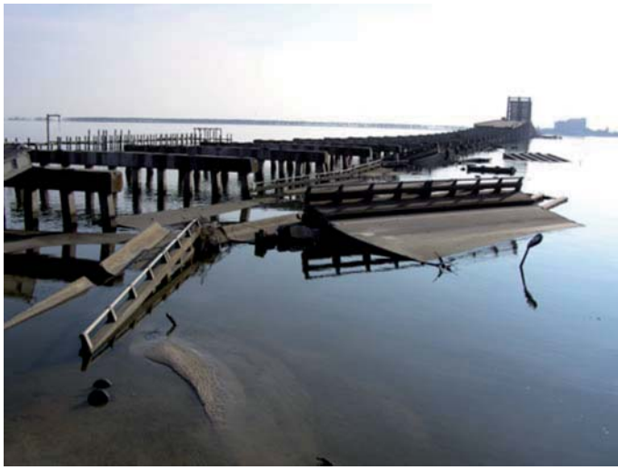
Figure 1. Deck damage on US90 bridge over Biloxi Bay.
