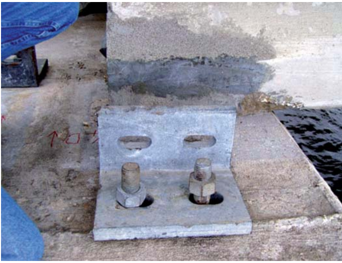
Figure 14. Anchor bolts missing from restraint angle.
