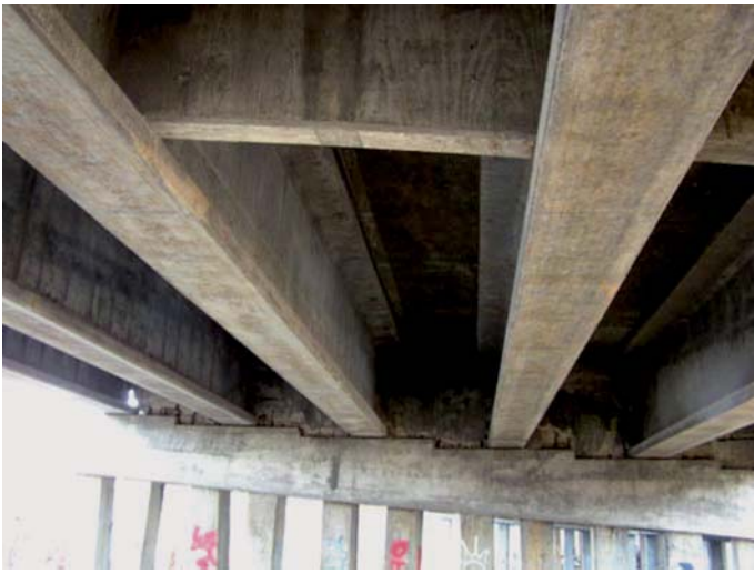
Figure 8. Soffit of US90 span showing potential trapped air volume.
